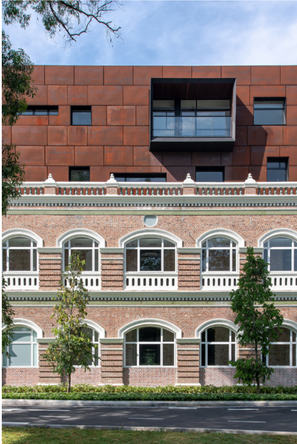
3rd floor front facade pop-out balcony (Relationship between the new and old)
